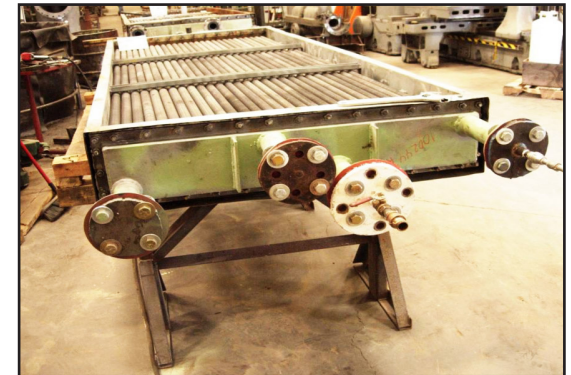
Unit being hydro-tested and readied for service.
