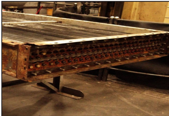
Corroded isophase cooler with rough and uneven surface.
